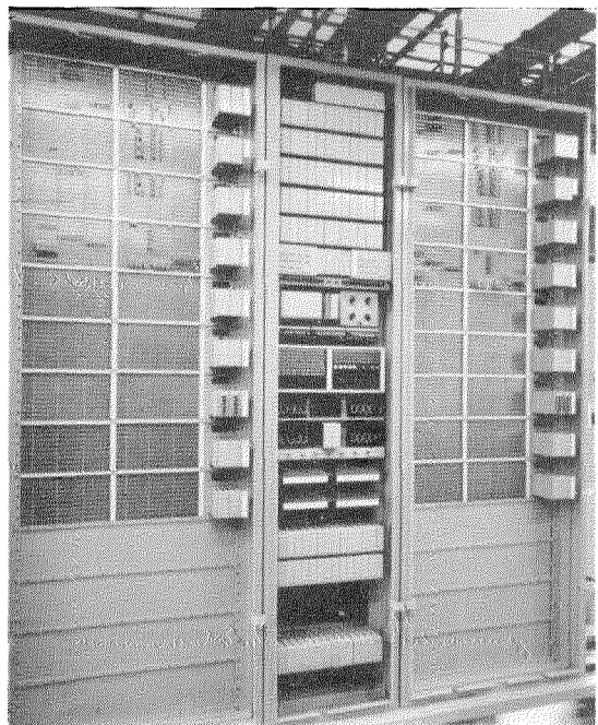
Figure 5—Installation of 2 translators and their common test equipment.
