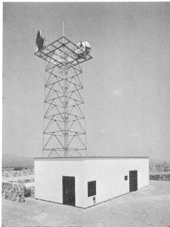
Figure 2—Standard unattended repeater station.
