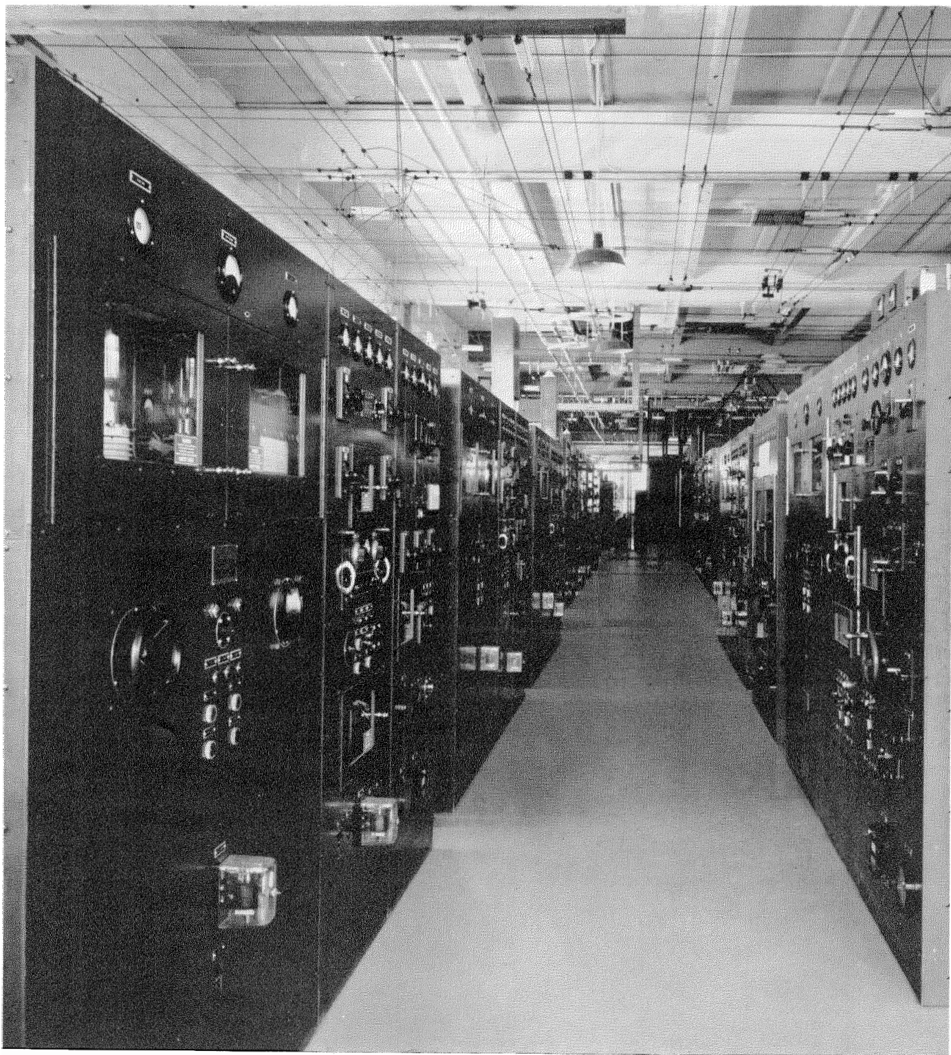
18. Two rows of high-power high-frequency transmitters at Brentwood. The grid of wires on the ceiling permits any of the 50 transmitters at the station to be connected to any of the outside transmission lines leading to the various antennas.
