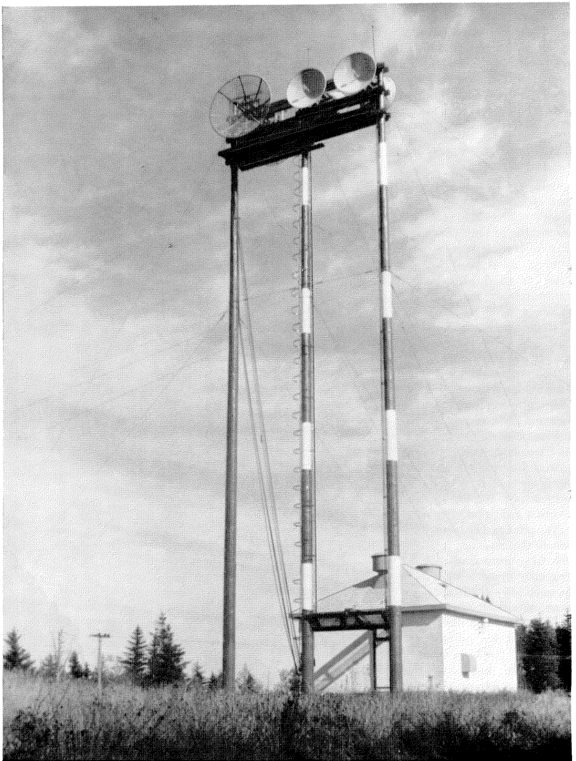
Figure 6—Repeater building and antenna arrangement at Upper Sackville.
