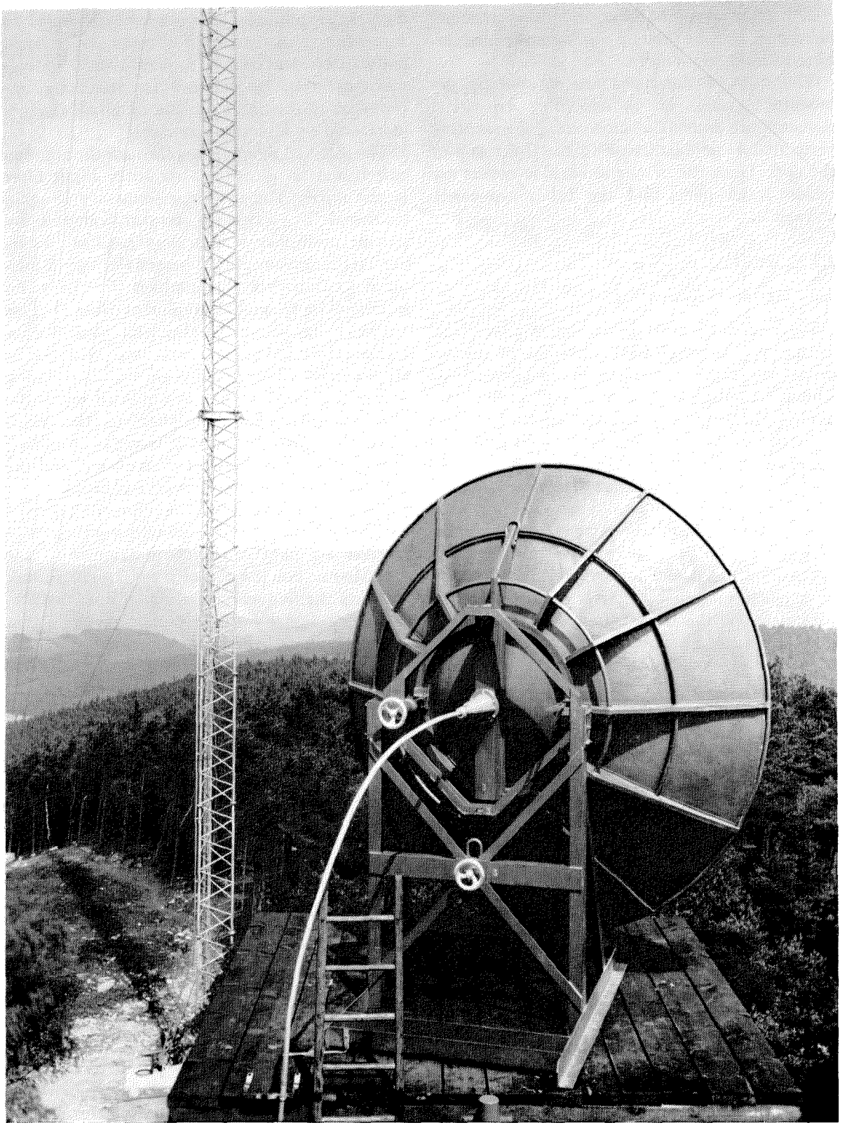
Figure 3—Paraboloidal antennas are used at all of the stations. They are 3 meters (9.8 feet) in diameter.
