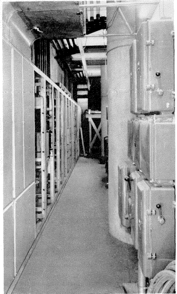
Figure 3—Rear view of power switchboard.
