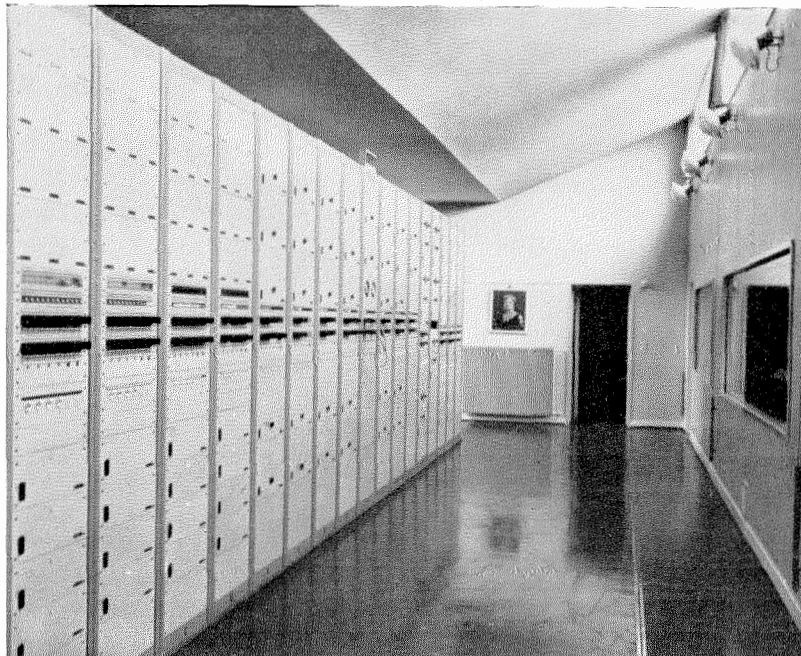
Fig. 2—Part of the amplifier room.
