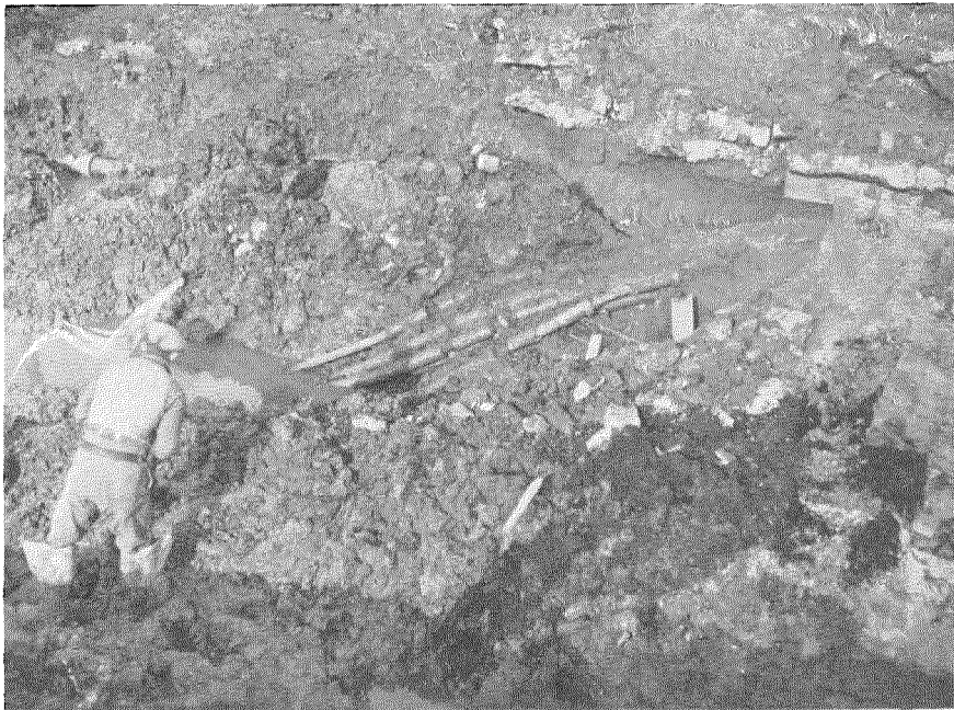
6600-volt power cable manufactured by S.T.C. uncovered in the London "blitz" continued in service. Sewage, gas, and water pipes nearby were all broken.
