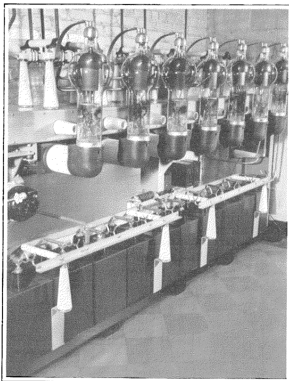
Fig. 11—Closeup of the 12-Kilovolt Rectifier Showing the Simplified, Clean-Cut Design Typical of the Entire Station.
