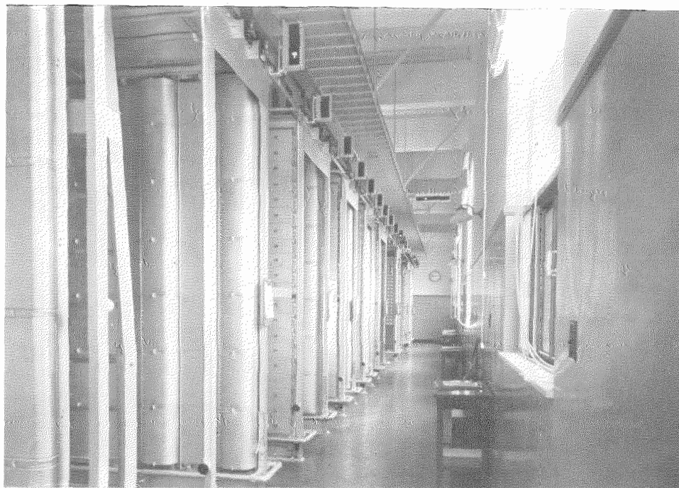
Fig. 7—An End Alley, Illustrating Cable Supports, Alarm Lamp Panels and Bay Dust-Shielding.
