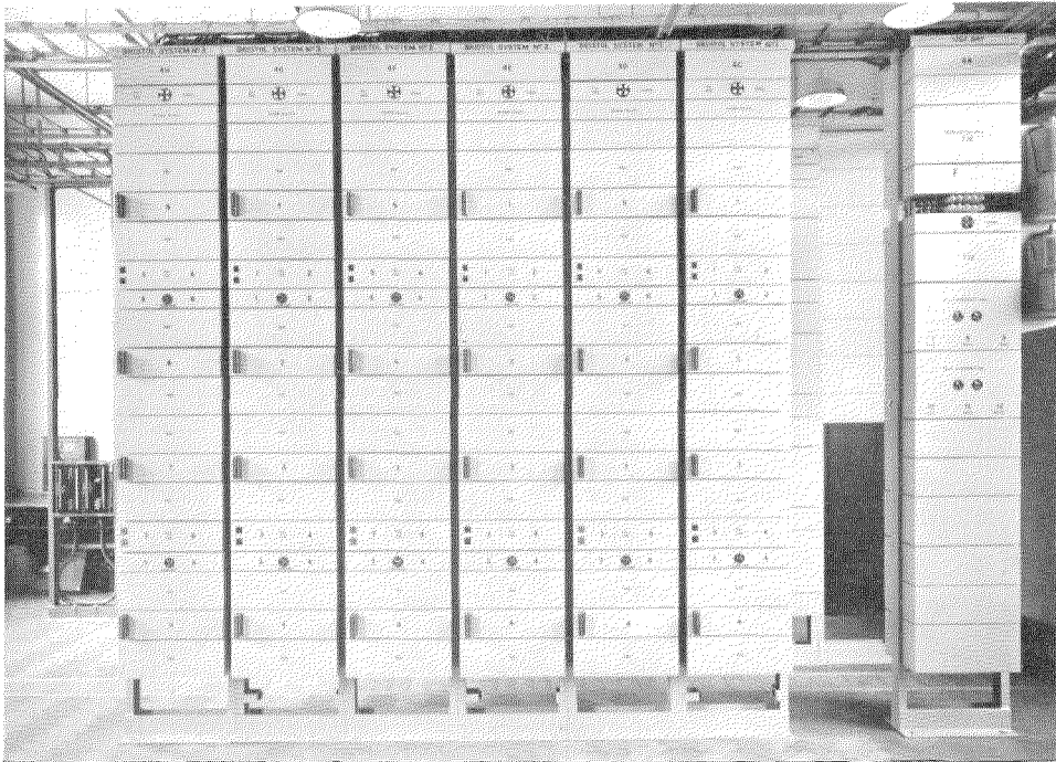
Fig. 5—General View of Terminal Equipment. One of first 12-channel carrier-on-cable installations, showing oscillator, channel and amplifier bays.
