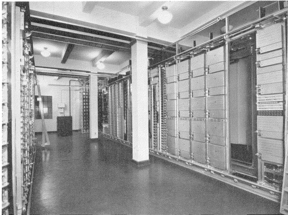
Fig. 3—7-A.2 Rotary Equipment in the Callao Exchange. Main Distributing Frame and Test Desk Are in the Rear.
