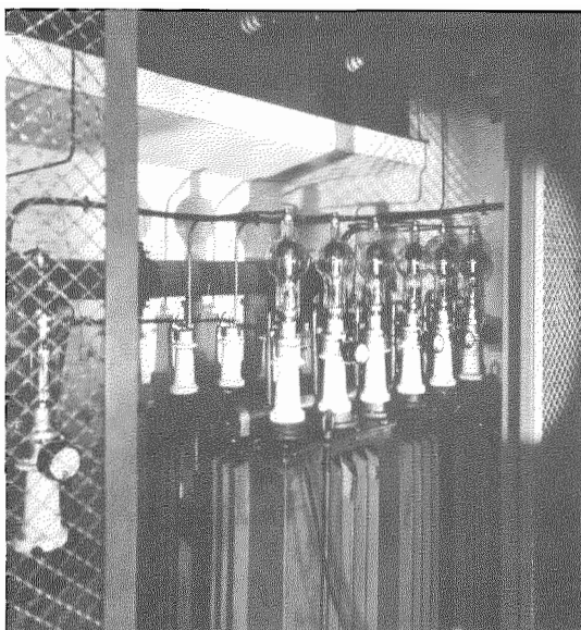
Fig. 17—One of the Hot Cathode Mercury Vapour Rectifier Units supplying the High Tension to the Power Stages of the Transmitter.
