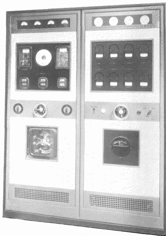
Fig. 19—Power and Water Control Board.
