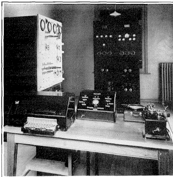
Figure 5—Traffic Room in St. Inglevert Building.
