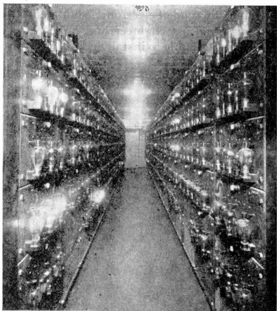
Fig. 3—One bank of electronic tubes controlling the lighting at Radio City Music Hall.
