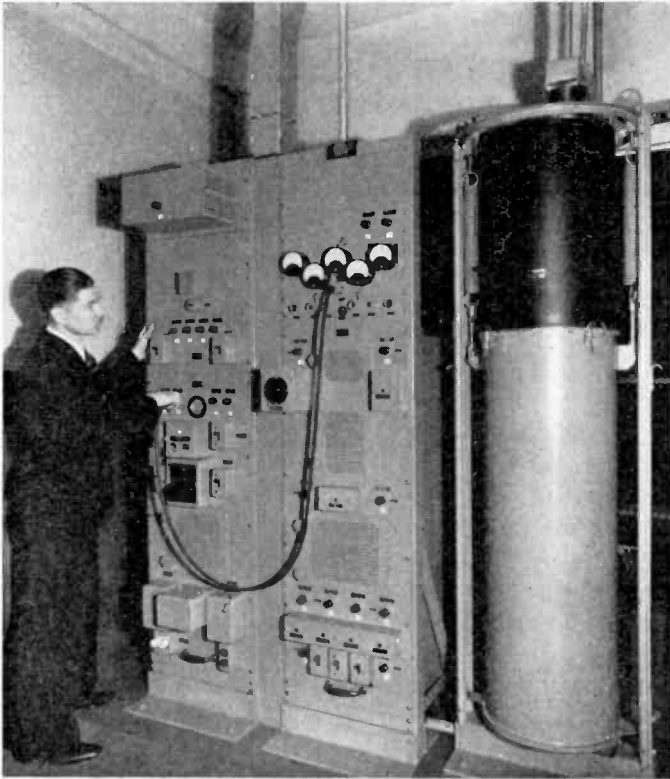
Fig. 1—Front view of an ultra-high-frequency transmitter (installed).
