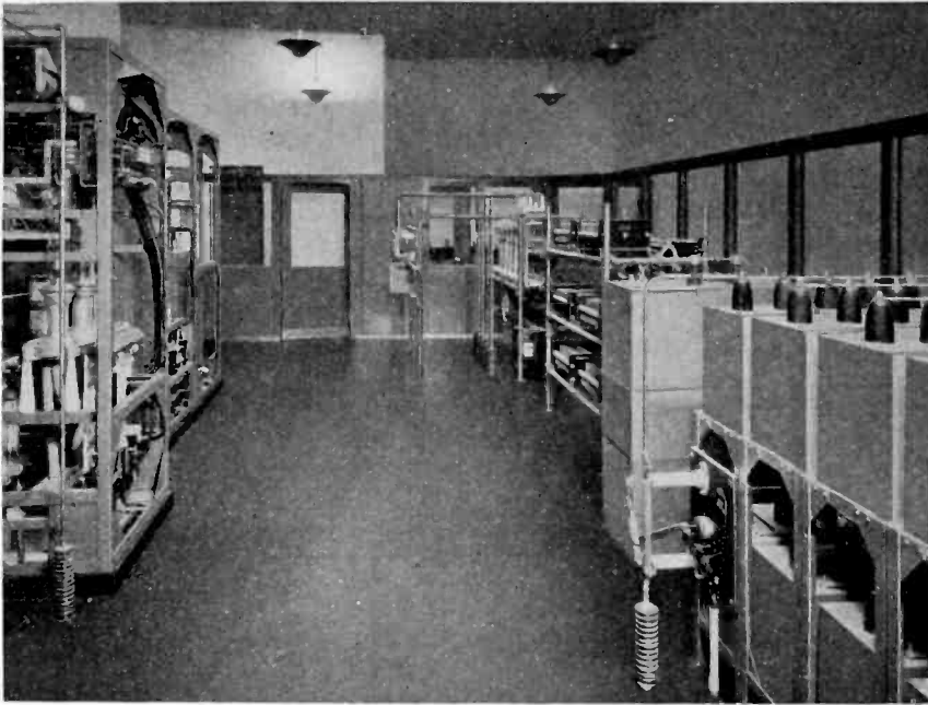
Fig. 9—Rear view of transmitter showing rectifier, switching unit, and high voltage filter.
