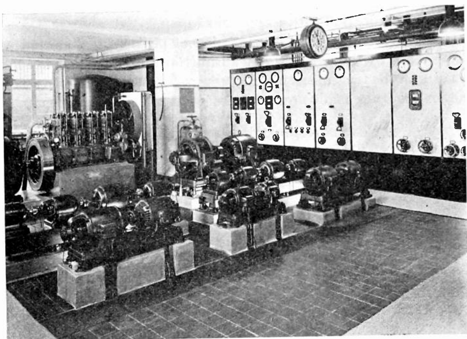
Fig. 21—Machine room of the Beelitz building for reception.
