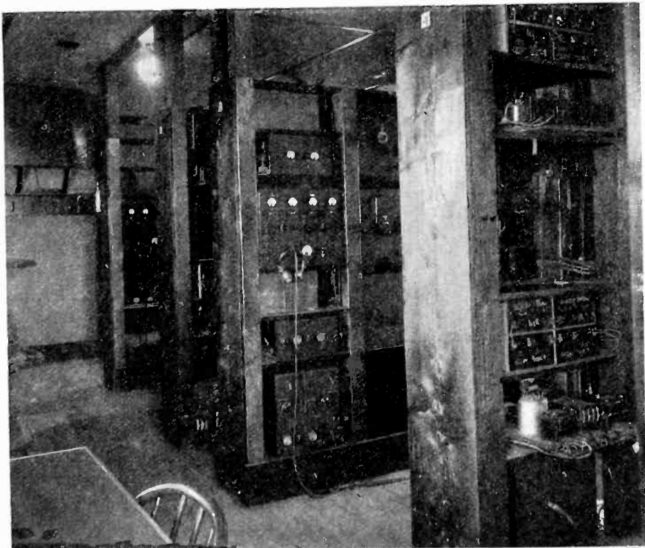
Fig. 19.—General view of racks in rebroadcast building.
