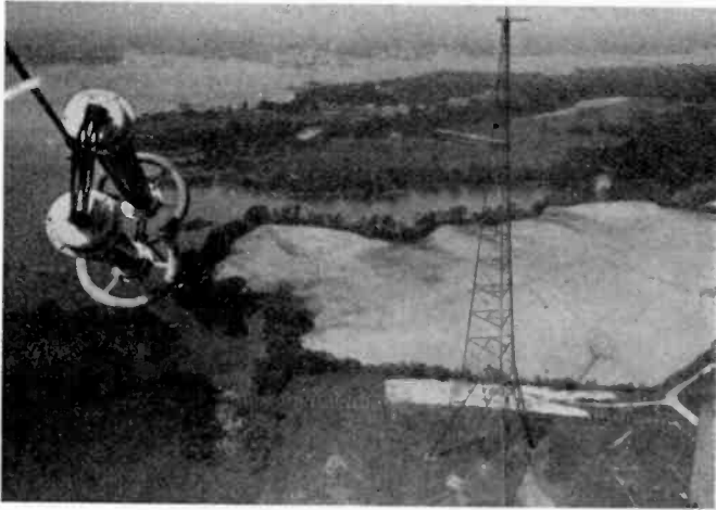
Annapolis, showing triatic insulator in position and suspension insulators on triatic number one viewed from top of tower.
