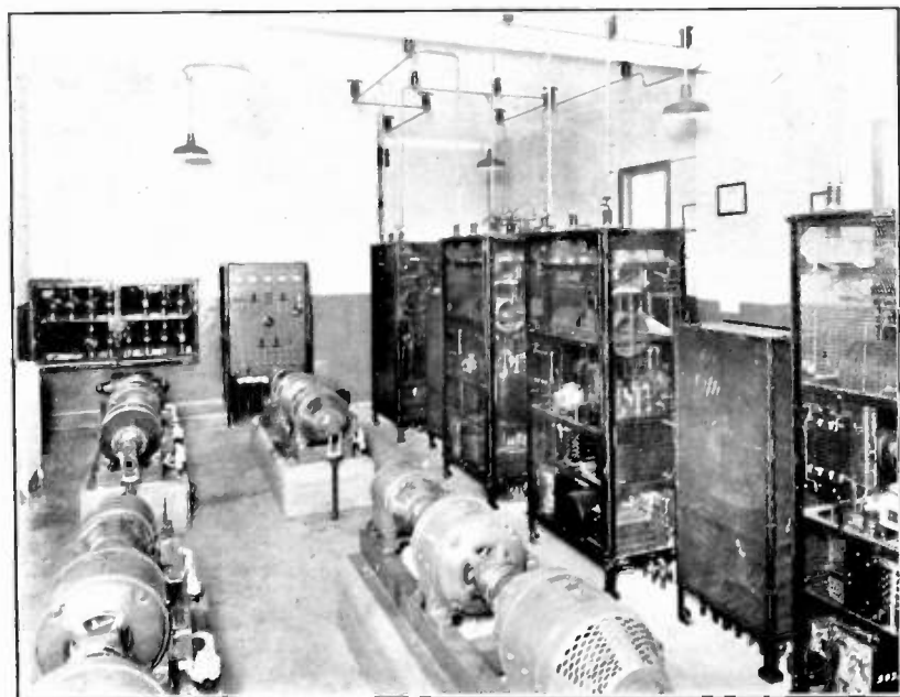
FIGURE 17—Transmitter House, Broadcast Central, Interior
