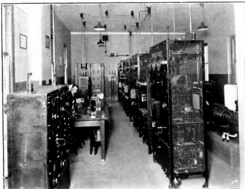
FIGURE 16—Transmitter House, Broadcast Central, Interior
