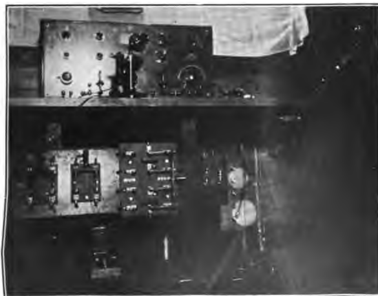
FIGURE 9—Receiving room at Ketchikan. On top of table, center is the 4000 meter marine tuner; on extreme right in corner is change over switch; underneath table is a wooden switchboard, mounted on which are: (starting at left,) a D.P. switch acting as two S.P. switches for disc and blower motors, 220 volt mains for converter, 4 pole starting switch, 5 K.W. rotary switch.
