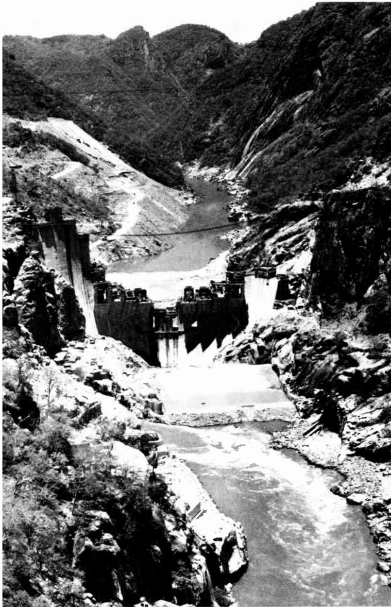
[1] A downstream view of the Cabora Bassa gorge of the Zambezi River in the northwest of Africa's Mozambique. This photograph was taken while the Cabora Bassa dam was under construction in November, 1973.
