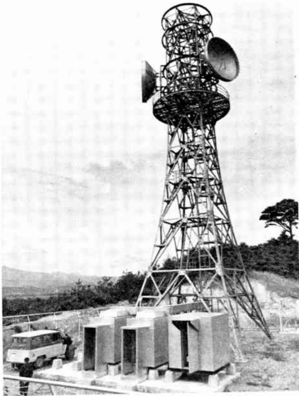
FIGURE 6. Example of an 11-GHz relay station housed in a small, transportable shed.
