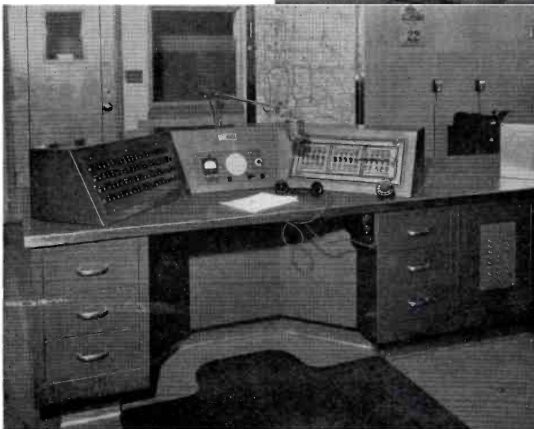
FIG. 5. THE POLICE RADIO SYSTEM CAN BE OPERATED FROM EACH ONE OF THE THREE CONSOLES
