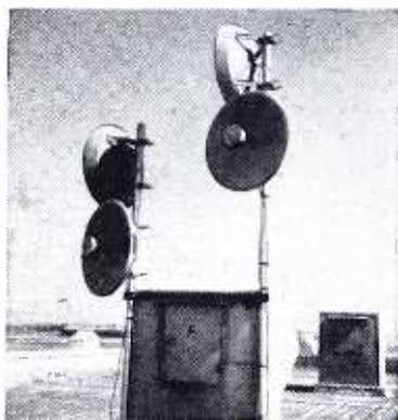
Two links of receiving and transmitting antennas of Central Arizona Light & Power Co., located on roof of generating plant.
