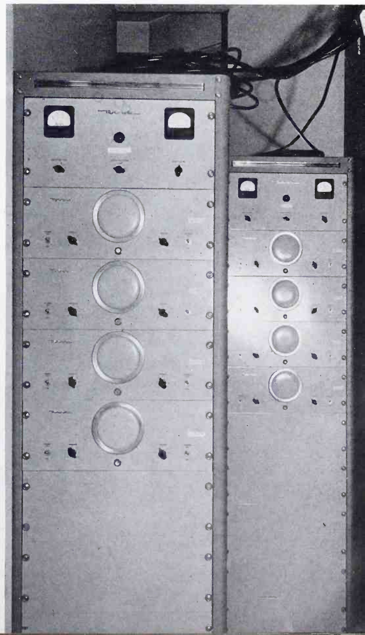
FIG. 6. RECEIVERS ARE LOCATED AT CITY HALL TO ELIMINATE MUTING DURING TRANSMISSIONS
