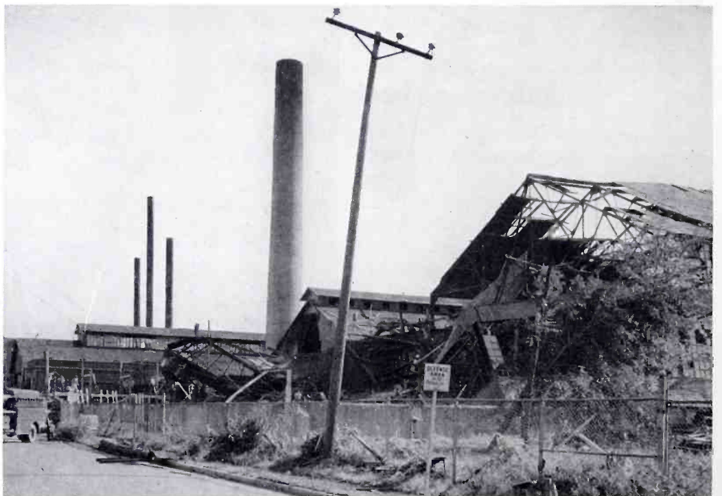
EXAMPLE OF TORNADO DAMAGE THAT PUT A PREMIUM VALUE ON RADIO COMMUNICATION SERVICE
