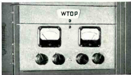
G-E Limiting Amplifier at the 50,000 watt transmitter of WTOP, Washington, D. C.
