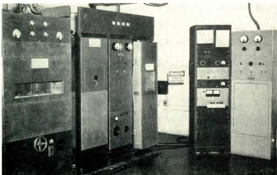
FIG. 5. THE COMPLETE 50-KW. TRANSMITTER BUILT FOR EXPERIMENTAL PURPOSES
