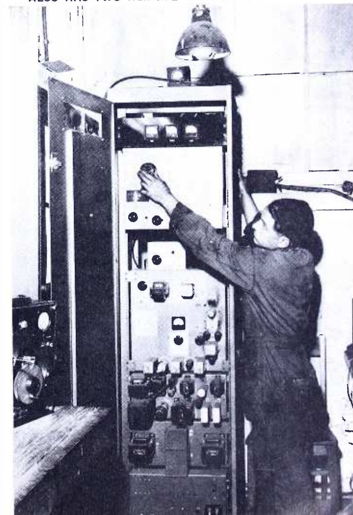
FIG. 3. TRANSMITTER-RECEIVER INSTALLATION AT THE MAIN GARAGE. SYSTEM ALSO HAS TWO REMOTE RECEIVERS
