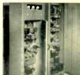
Equipment at Mt. Caalidge. Left, Motorola beam transmitter and receiver. Right, Motorola 250-W. transmitter and receivers.
