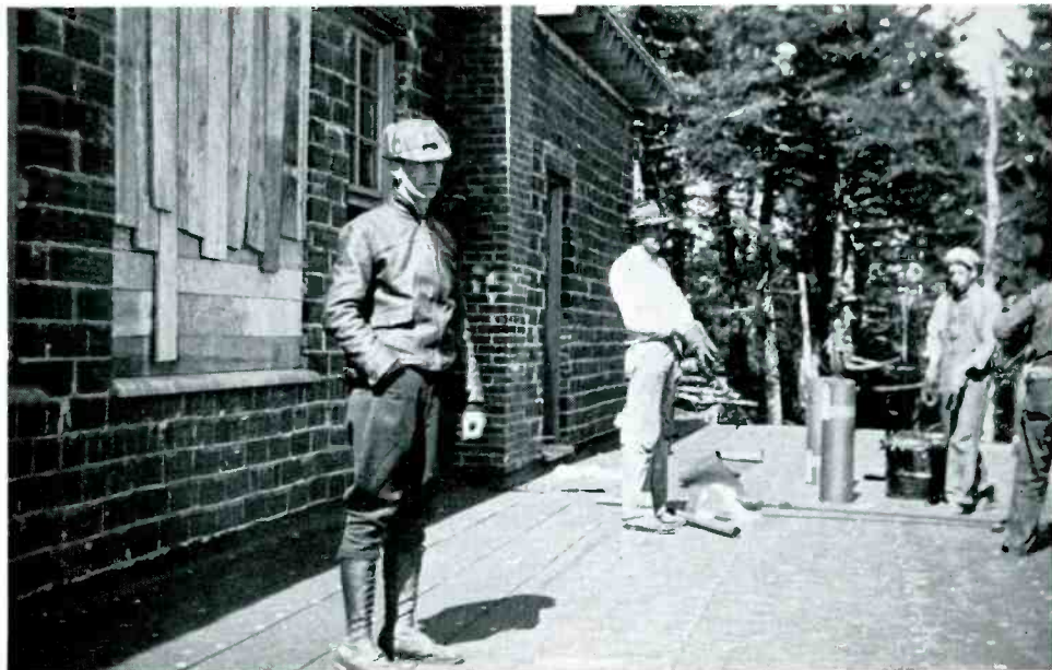
THE AUTHOR, LEFT, STANDING ON THE ROOF OVER THE LIVING QUARTERS. THIS WILL BE AN OBSERVATION TERRACE FOR VISITORS. THEY WILL LOOK INTO THE TRANSMITTER ROOM THROUGH A WINDOW
