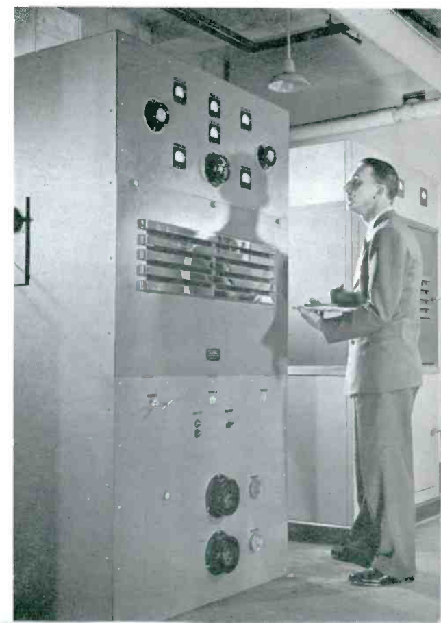
FIG. 4. LEFT, THE 50 KW. POWER AMPLIFIER STAGE. AT THE RIGHT IS THE HIGH-VOLTAGE RECTIFIER
