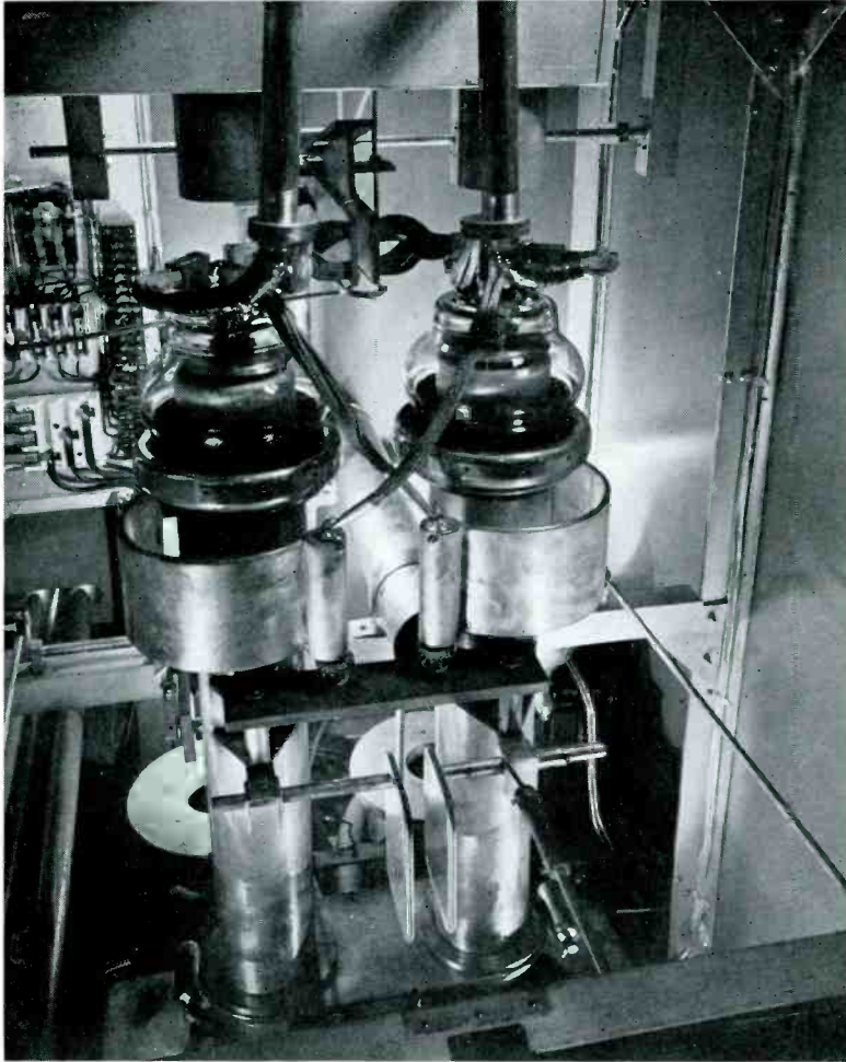
FIG. 6. FINAL STAGE, WITH THE GL-880'S, AS SEEN FROM THE FRONT OF THE CABINET
