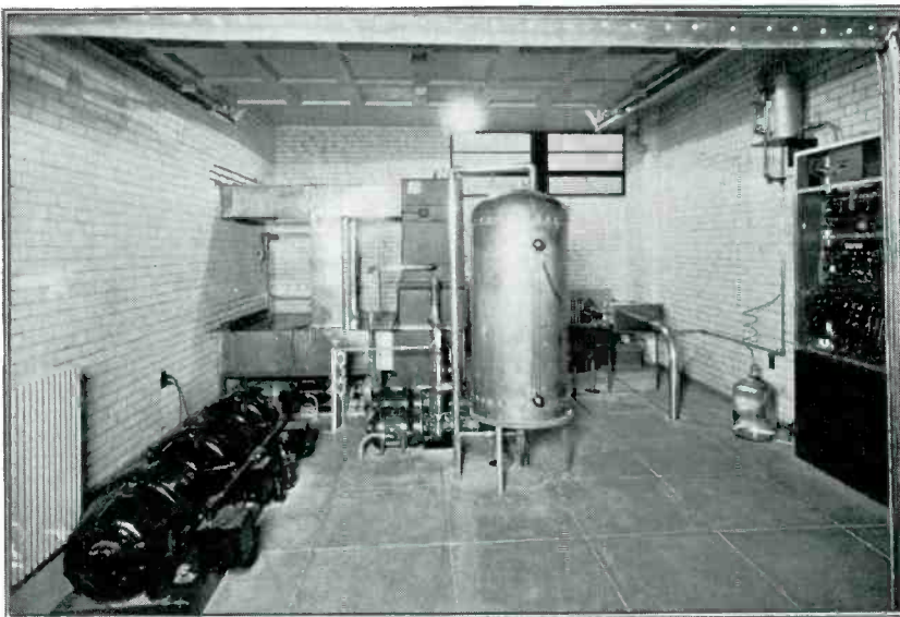
FIG. 9. THIS ARRANGEMENT AT PAXTON, MASS. IS SIMILAR TO W55M LAYOUT, SHOWN IN FIG. 7
