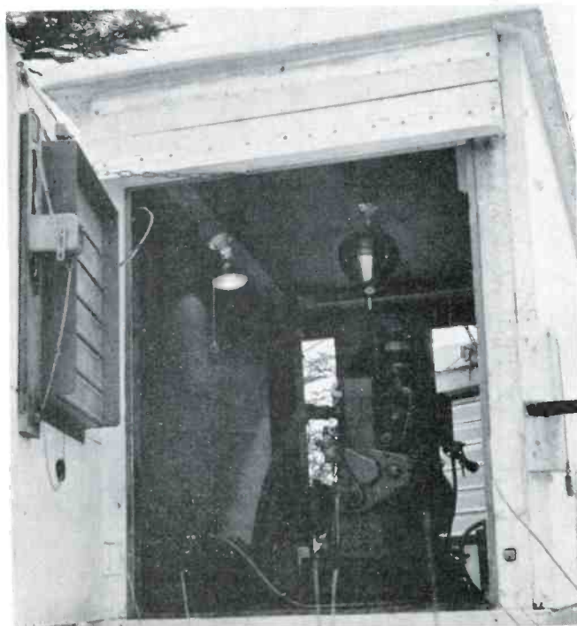
FIG. 6. VIEW OF GENERATOR SHACK THAT SHOWS VENTILATING LOUVRES
