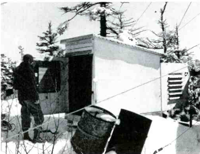
FIG. 5. EMERGENCY GENERATOR SHACK IS BUILT ON STILTS FOR WINTER
