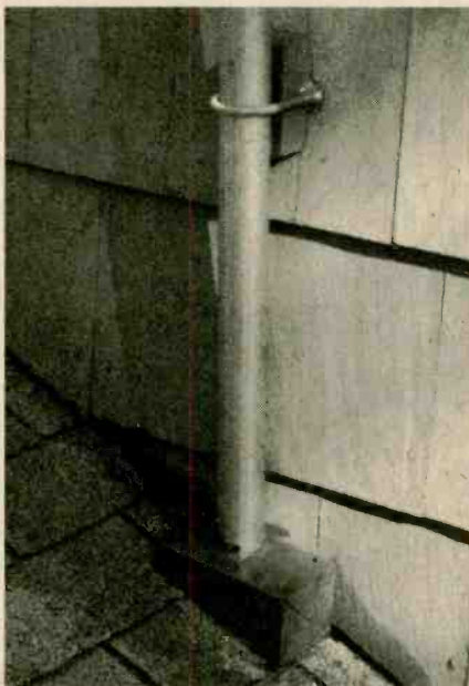
Bottom of antenna mast fits into hole drilled part way through a wedge-shaped block protecting roof shingles. U-bolts pass through wall of house into attic. Note spacer block between the mast and wall to keep the mast vertical.
