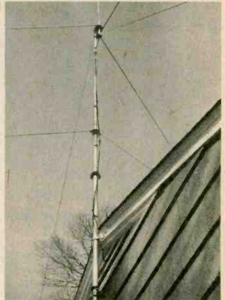
Telescoping mast can be lowered in minutes without disconnecting guy wires, to bring the antenna within reach for maintenance and troubleshooting.
