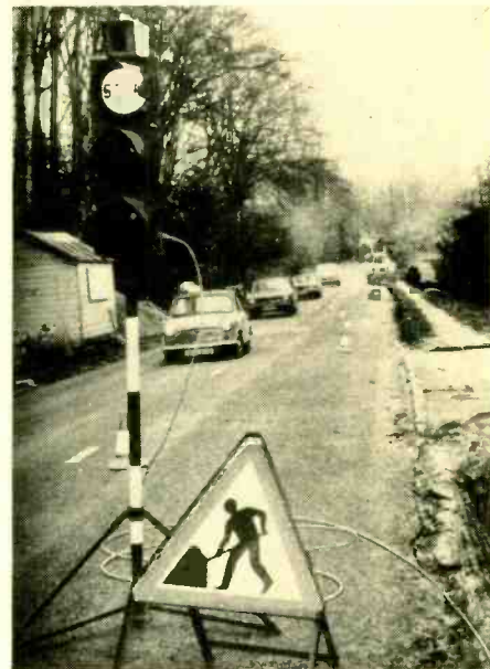
Taking power from a nearby street lamp or power main, the radar-controlled traffic light controls two-way traffic in one lane.
