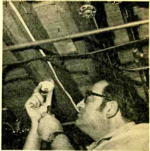
Standard open circuit heat/fire detectors can be installed in all living areas, above the furnace and in cellar and attic.
