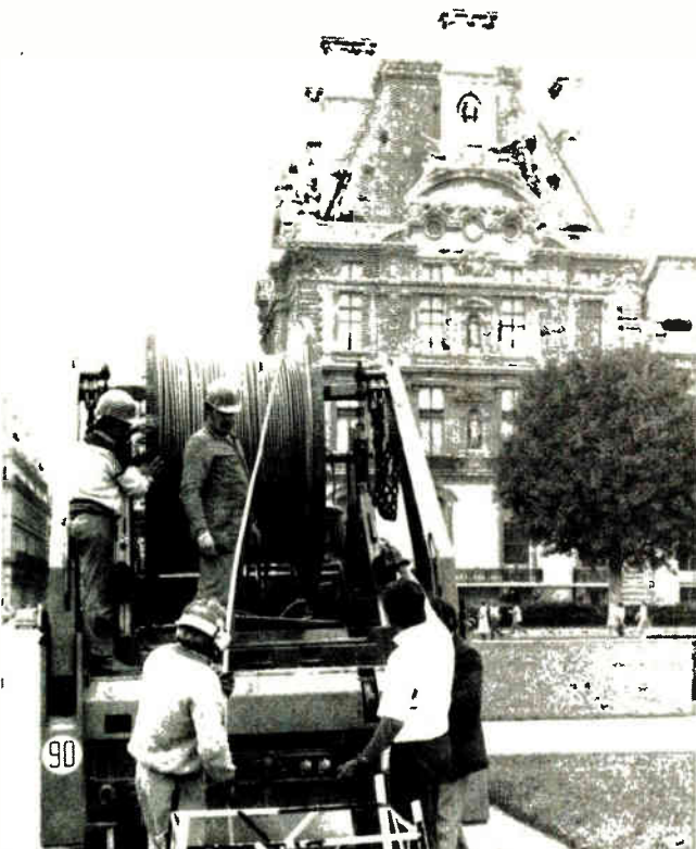
Past meets future. In the Tuileries garden of the Louvre palace in Paris, workmen install a high-capacity 7-kilometer fiber-optic line linking two exchanges in the central portion of the city. While such links are not yet much of a market, their day will soon come.
