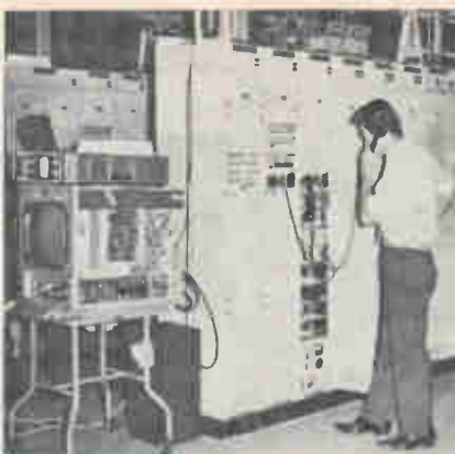
Key element. Carrier signal center in communications tower is an integral part of Mexico's new microwave net.
