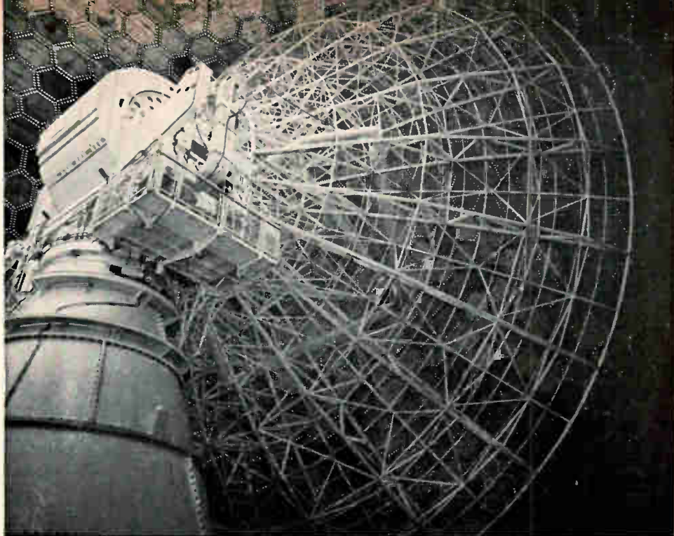
The 84-foot parabolic antenna is protected from the severe Alaskan winters by a radome 140 feet in diameter. The antenna and pedestal weigh 200 tons.
