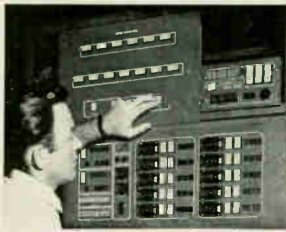
Whittaker control unit consists of monitor panel, top left, master control panel, right, and decoder box at bottom.
