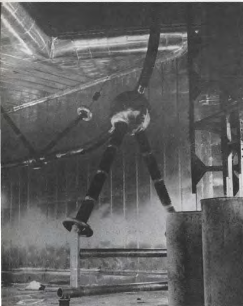
Anticorona fittings applied to the high-voltage trunk at Navy radio station in Cutler, Me. The room is copper-shielded to prevent eddy currents in building structure.
