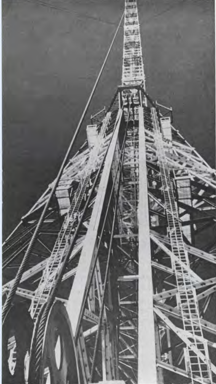
In the foreground a counterweight track of the Cutler, Me. vlf antenna system. The antenna tower, separate from the track, is in the near background. (Continental Electronics Mfg. Co.)
