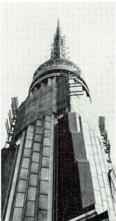
TRANSMITTING antennas atop Empire State Building
