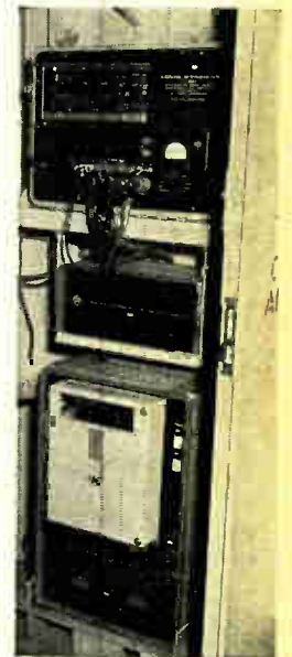
Clock, control unit, and recorder mounted in the Gyro Room of the Mormacpride's Bridge Deck.
