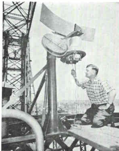
Raytheon radar atop vertical lift bridge at Duluth, Minn., warns of approaching ships in heavy weather
