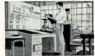
3. Instrumentation, control, and switching systems
