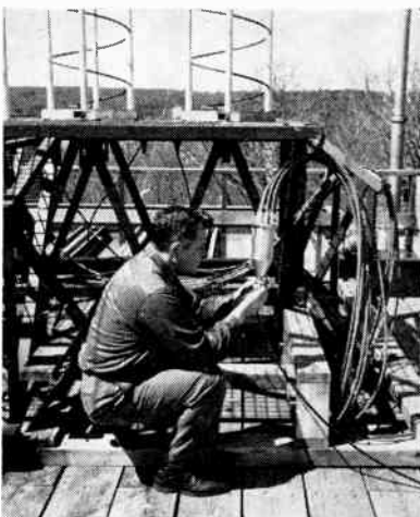
Cables here shown being connected to power divider, lead to elements in helical antenna array
