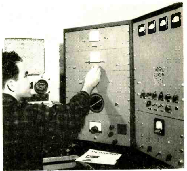
Operator is shown adjusting plate current of uhf converter r-f amplifier to optimum level. Front panel contains 0-50 ma meter and switch that provides check for each 416B r-f amplifier
