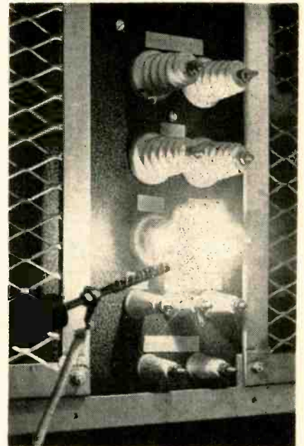
Photograph shows the results of a short-circuit at 5,000-volt operation. Here the fault protector was not incorporated as a part of the circuit
