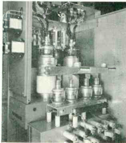
Center cubical of GATES HF-10 Transmitter illustrates husky tank circuit design for high efficiency coverage over entire frequency range.
