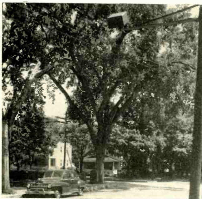
Typical radar traffic-control installation shows equipment mounted on long bracket over street. Echoes from approaching cars keep traffic signal green
